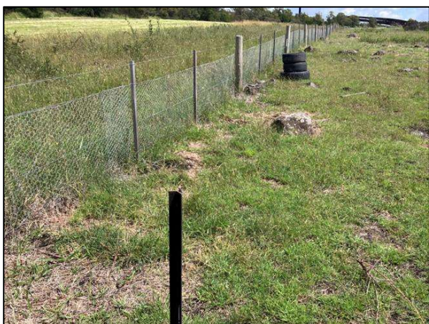
Plate 25. Good condition perimeter fencing along the western boundary (Ecology and heritage Partners 01/12/2025).
