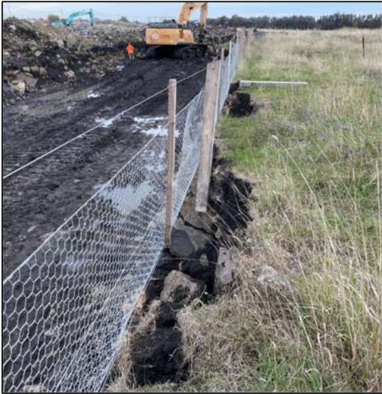
Plate 39. Erosion of offset site adjoining construction area during Year 1 (Ecology and Heritage Partners Pty Ltd 31/05/2023).
